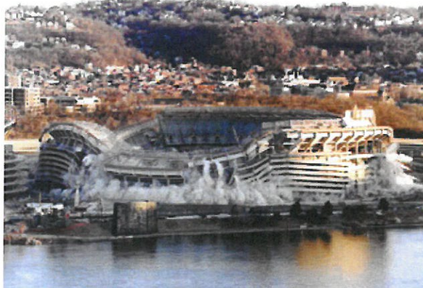
Demolition of Three Rivers Stadium & Engineering Services for Heinz Field Pittsburgh, PA
